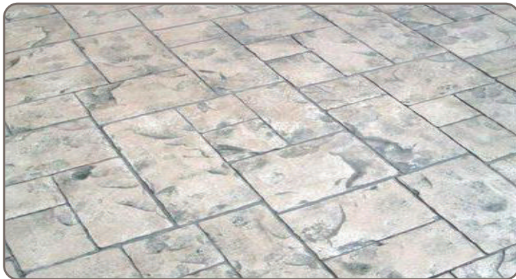
BEFORE: Old, faded, worn stamped concrete.
